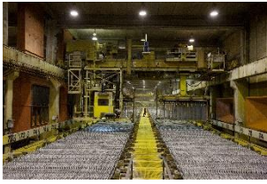
Zinc cell house
